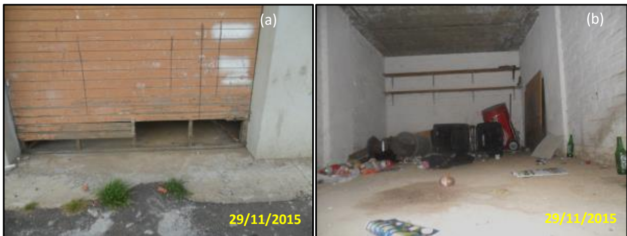
Figure 5: (a) Broken garage door at the Da Gama Park Naval Flats. (b) Inside the garage after it had been raided by the baboons.
